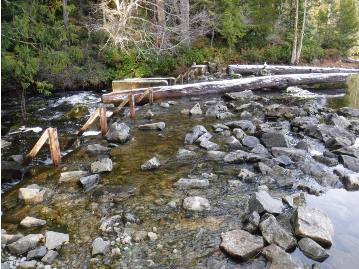
Photo 2: Upstream area of the dam and jammed logs
