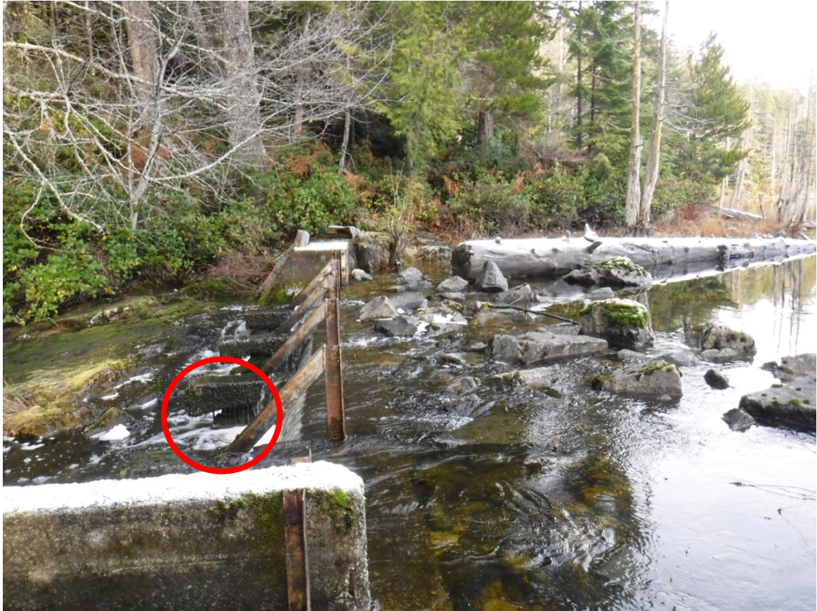
Photo 3: Downstream area of the dam and undermined foundations
