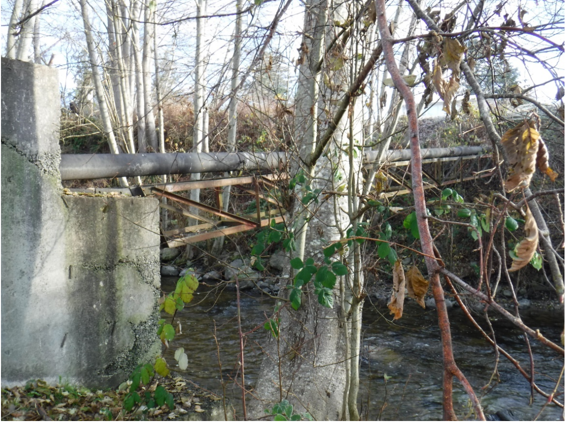
Photo 7: Wastewater treatment plant piping
