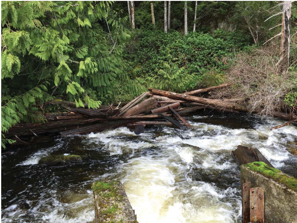
Figure 7 – Jammed debris material and logs downstream of the weir dam
