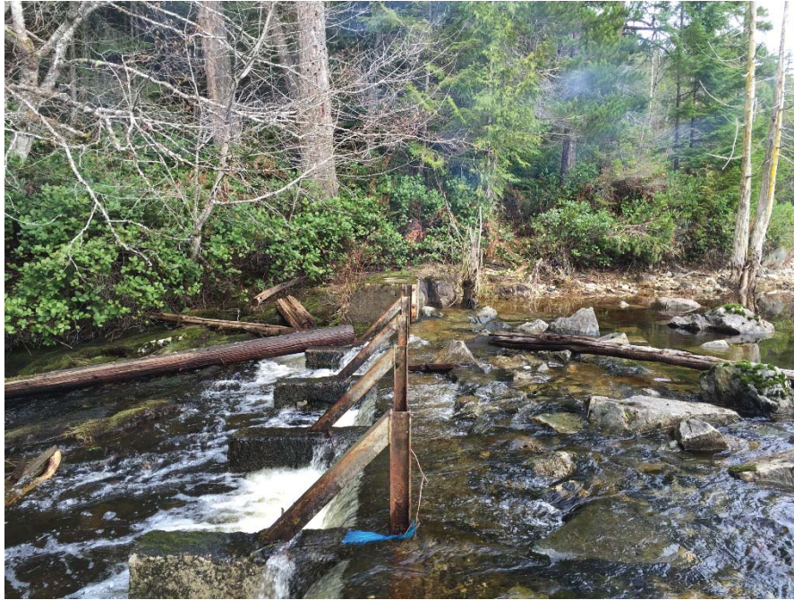
Figure 8 – Debris and erosion evidence on the right abutment of the weir dam
