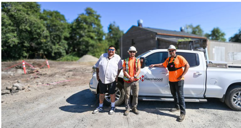
Tla'amin Nation hegus John Hackett, Daniel Girard, Hazelwood Superintendent and Brandon Huddleston, Hazelwood Foreman at the site of the soon to be decommissioned sewage treatment plant
