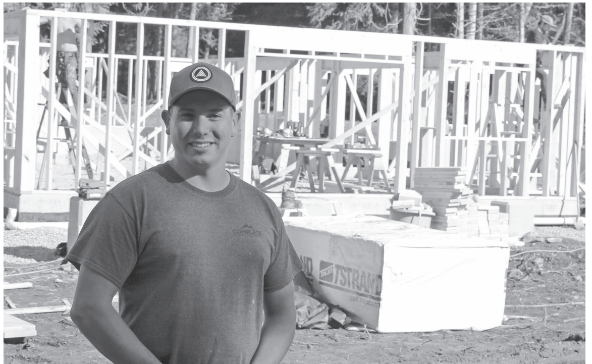
Craig Galligos is proud to be working for his nation at the Klahanie subdivision
