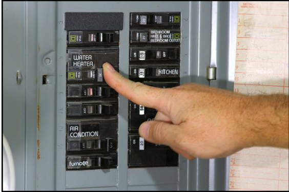
Hot water shut-off on breaker panel
