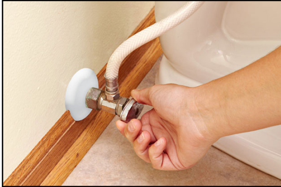
Water shut-off at back of toilet
