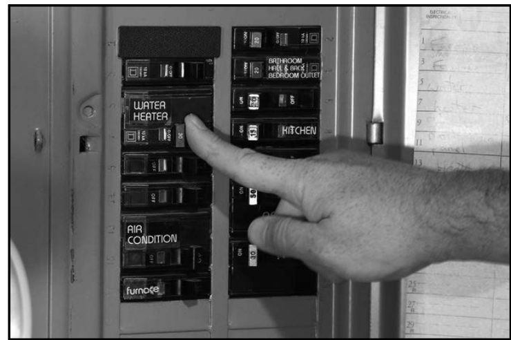
Hot water shut-off on breaker panel
