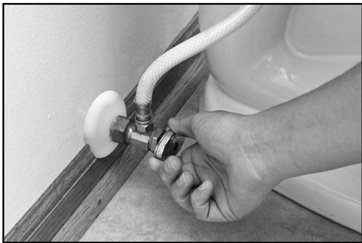
Water shut-off at back of toilet
