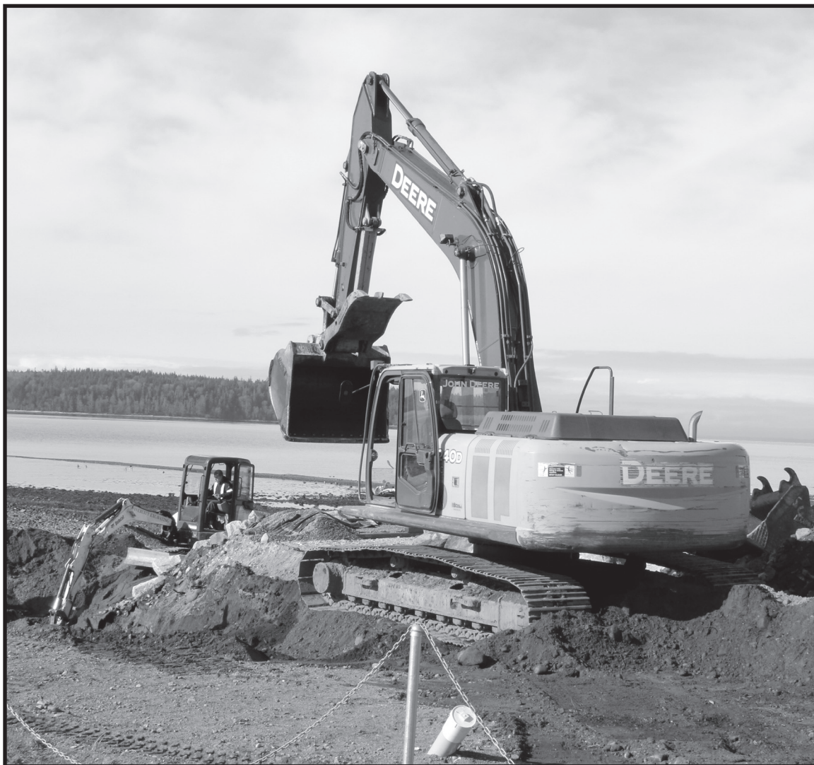
An old waterpipe has been causing problems for the outflow and is replaced
