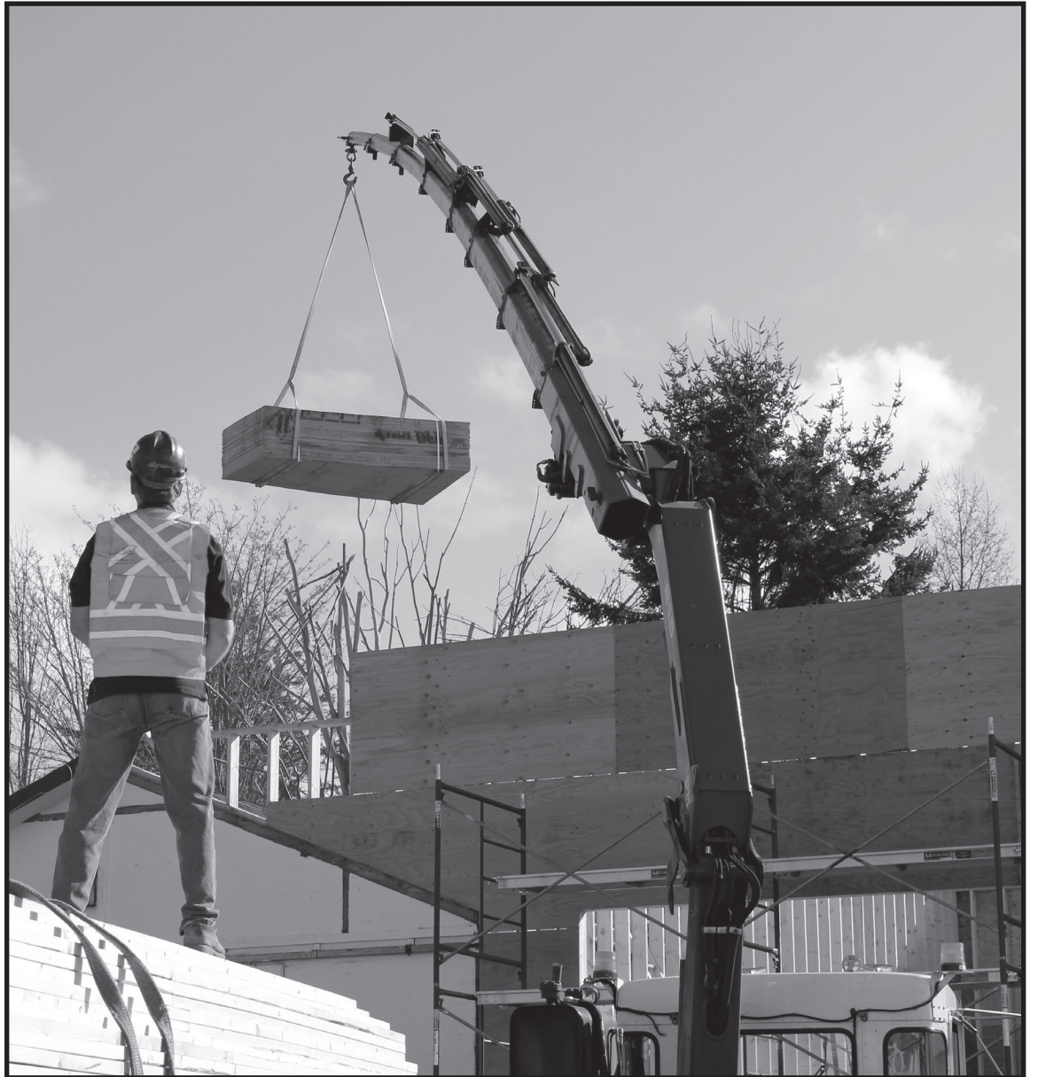
Our firehall is getting renovated to make room for a second firetruck
